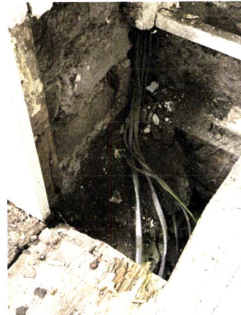
Damp from chimney and ground.
