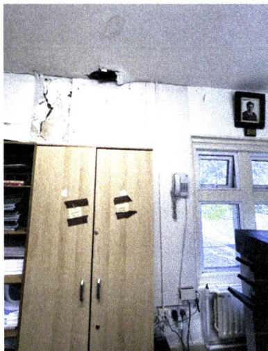
Teacher's Room Water ingress from Valley over.
