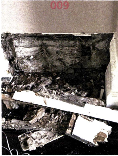
Skirting Board Dry Rot
