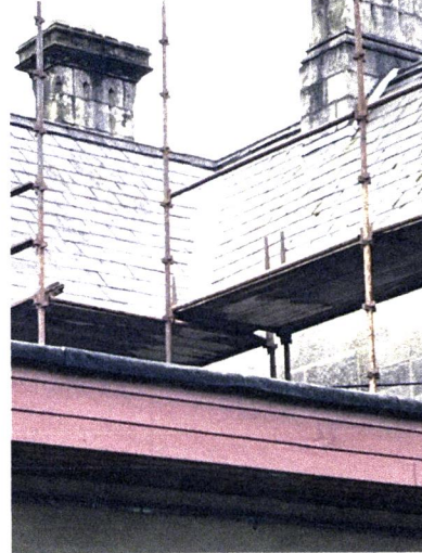
Valley repaired. Boards, lead and slate replaced. Cast iron rainwater gutter - profile special order.
