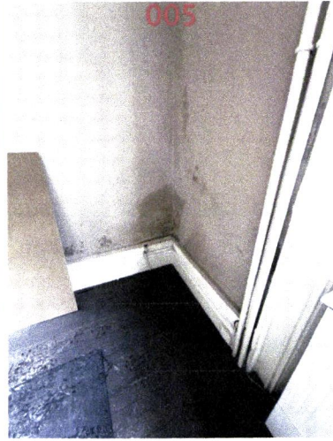
Damp corner of Room.
