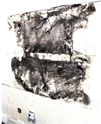
Manager's Room - Wet Rot identified. Concealed window on rhs of Rot.
