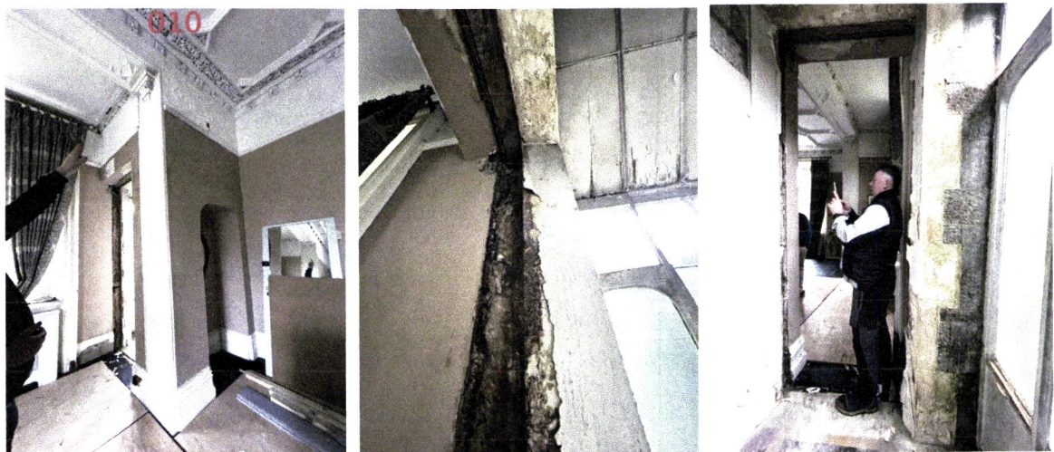
Door Removed revealing dense Dry Rot infestation behind door frame.
