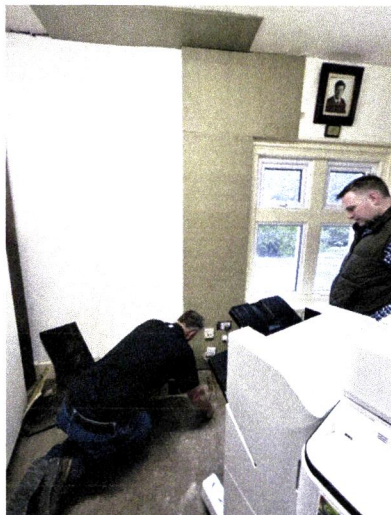
Teacher's Room - Wet Rot identified.
