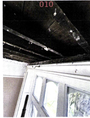
Bay window flat roof joists rotten.
