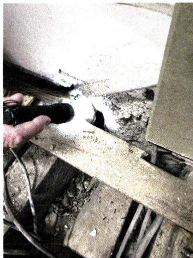
Floor joists under valley now repaired - rotten in wall Floor springy - localised rotten timbers.
