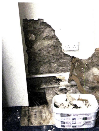
Opened-up floor joists rotten.
