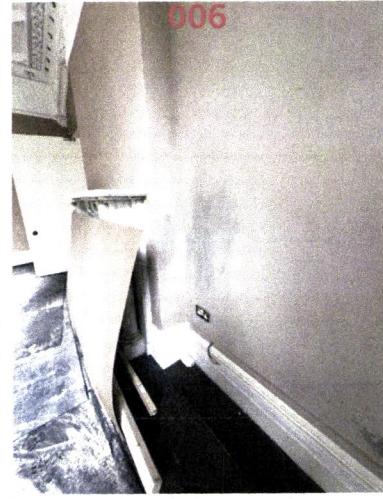
Damp at rhs of Chimney breast.
